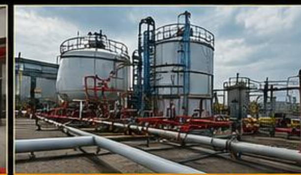
LPG TANK FARM PROTECTION
