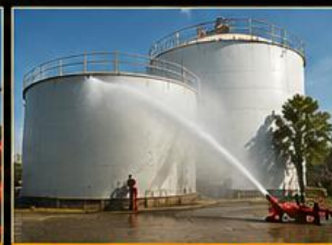
DELUGE SYSTEM IN ACTION
