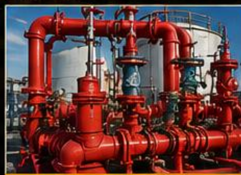
FIRE PUMP SYSTEMS
